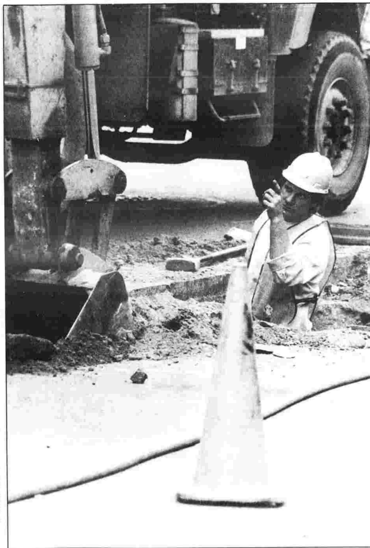
CREATING COMMUNICATIONS — John Conway, a town worker subcontracted by Southern New England Telephone, installs phone lines at the intersection of Broad and Center Streets in Manchester.
